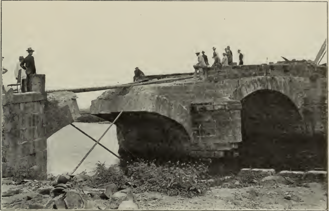
BRIDGE NEAR CALOOCAN ; THE ARCH, DESTROYED BY DYNAMITE BY THE INSURGENTS, IS BEING REPAIRED BY THE ENGINEERS.
